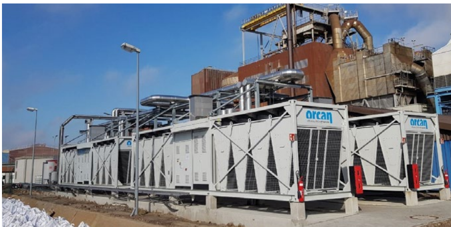
Four Orcan efficiency PACKs connected to the Nordenhamer Zinkhütte GmbH roasting plant, where they produce over 5,000 MWh of electricity per year from surplus heat.
