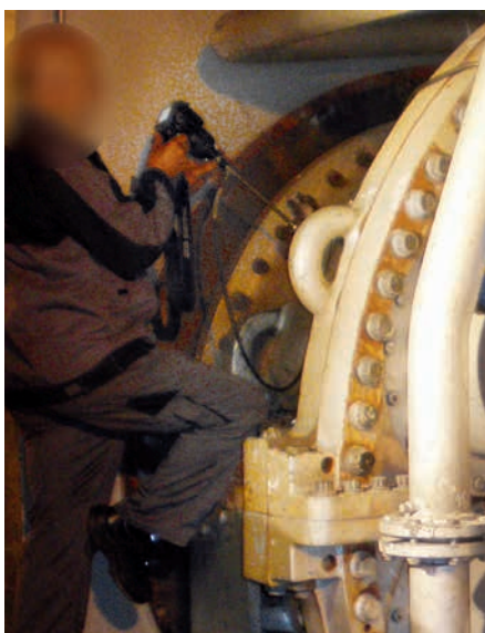
Gas turbine being inspected for damage by a boroscope (endoscope).
