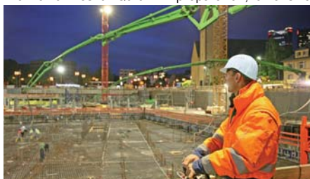
Putzmeister truck-mounted concrete pumps in action to construct the Frankfurt Telecommunications Tower.
